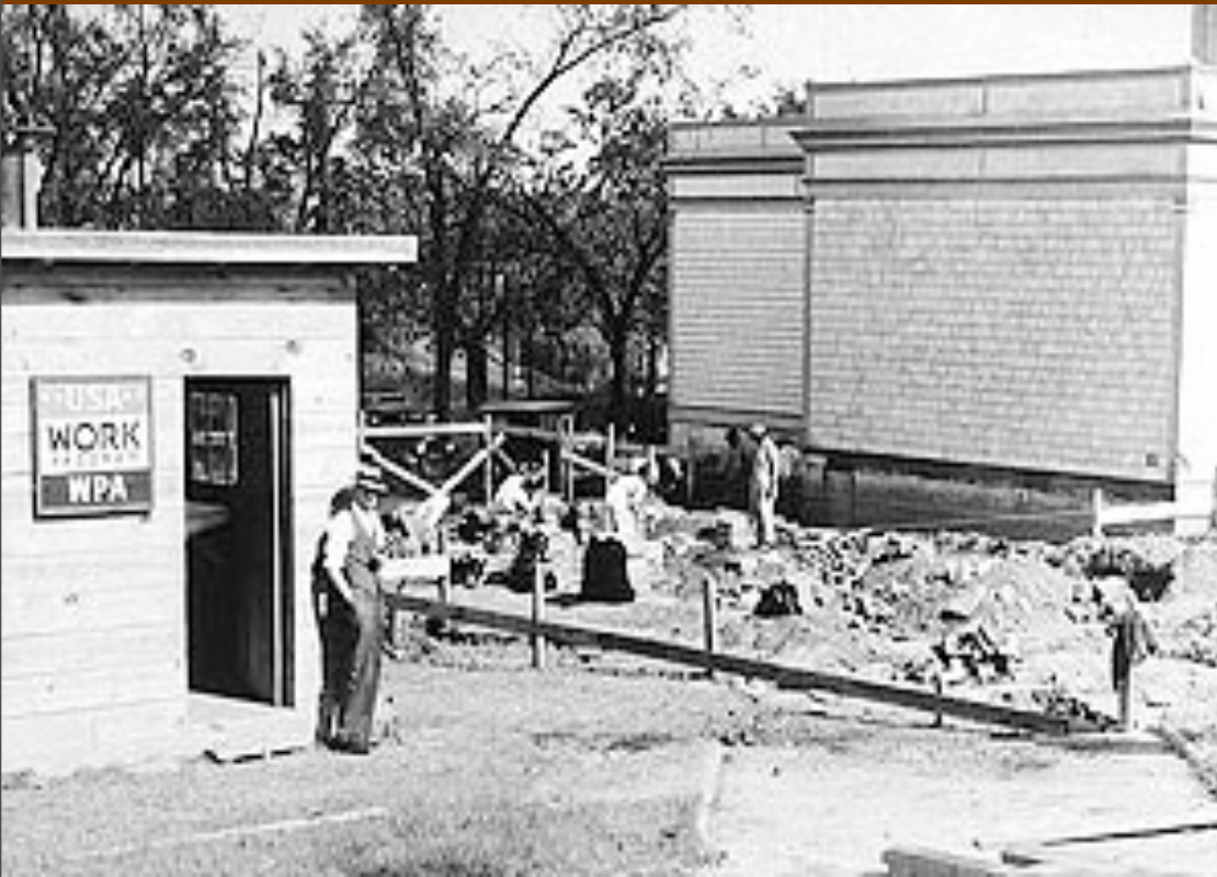
The Davis Street School Extension in Atlanta under construction as part of the Works Progress Administration Program, November 2, 1936
